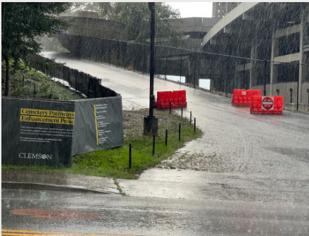
Press Road (beside Woodland Cemetery) is temporarily closed to non-service vehicles due to construction in the area. Photograph by Marquise Drayton.
