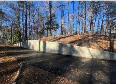
Retaining wall on the southeast side of the cemetery at Clemson University. Photograph by Marquise Drayton.
